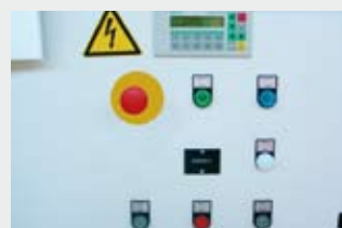
Stored-program controller PLC, operator panel with display.
